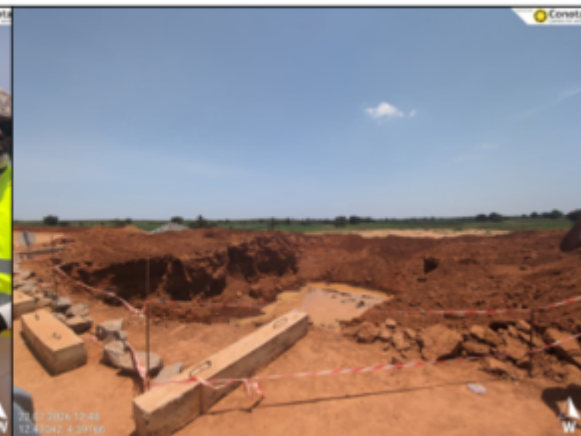
Photo 6: Dug up area with standing water
