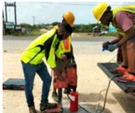
Coring of asphalt to check for the density and thickness of asphalt
