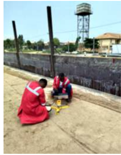
Field density test to determine the relative density of the compacted soil. The relative density is measured by comparing maximum dry density from field test with maximum dry density of laboratory test as standard reference
